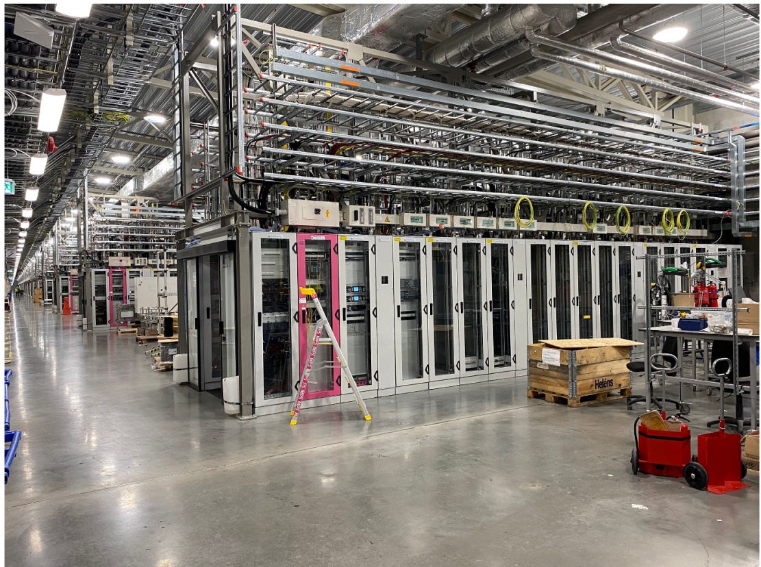
Figure 5. Control racks at ESS. Some racks are empty since the high energy end of the accelerator, from where the picture is taken, has not yet been installed. The image gives an impression of the size of control systems at accelerator-based research facilities.
