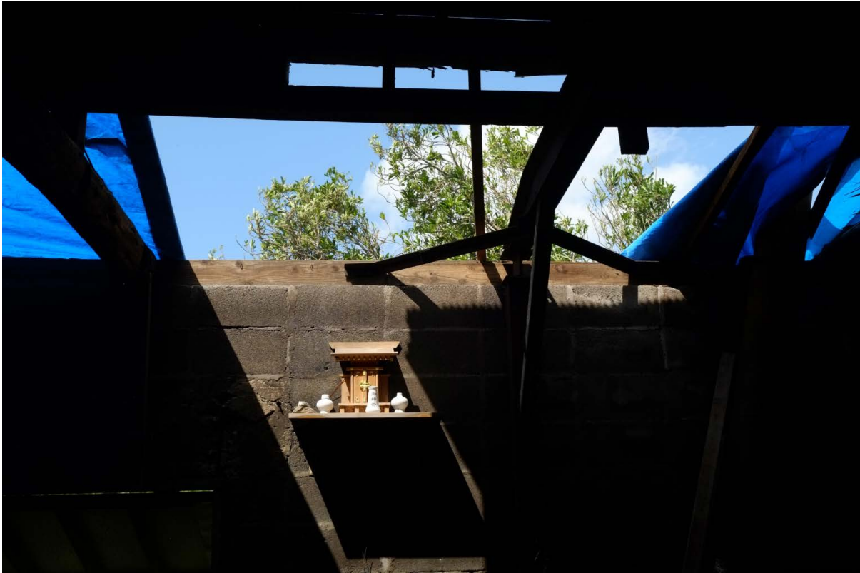
After a strong typhoon the doro workshop lost its roof, but the kamidana was mostly untouched.
