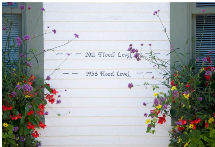
Figure 42. Flood marker, Wilmington, VT, now also featuring Hurricane Irene [Photo: Author 2103]
