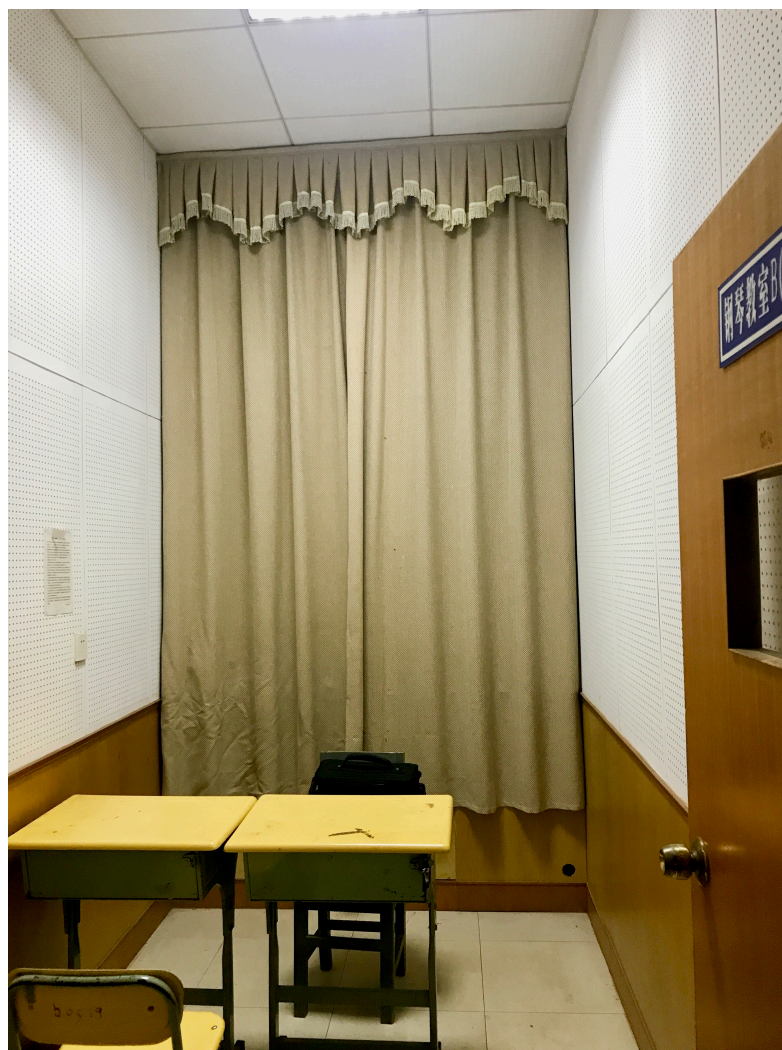
Figure 3.2: The music room with porous sound-absorbing wall materials for sound recording in Changsha Nanya Middle School, Hunan, China. On the door, it says Piano Room B .
