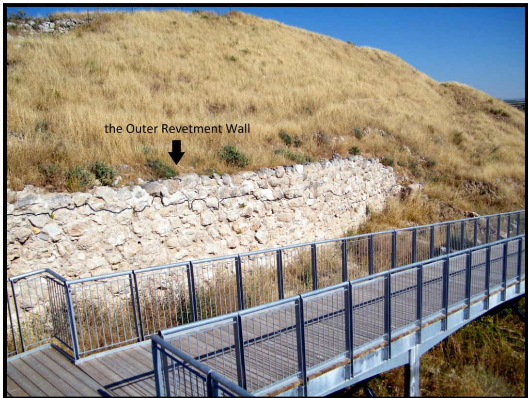
Fig. 17 (top) Black-painted cement lines at the bottom of the reconstructed western wall of the “guardroom” and beside the drain, view east; (bottom) a black-painted cement line along the reconstructed Outer Revetment Wall, view south-east (Photos: A. Zammit).
