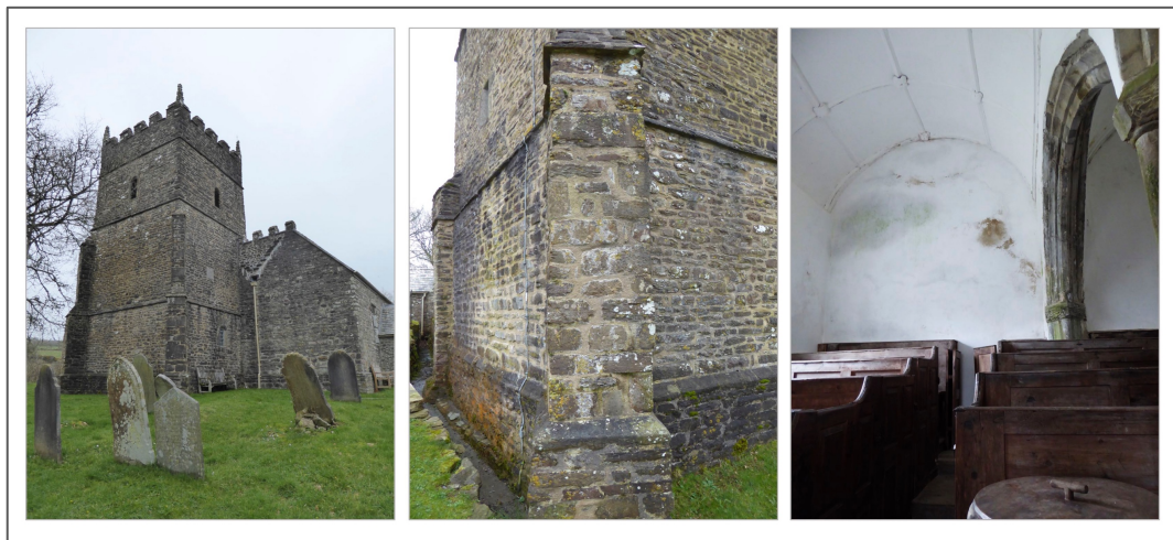
Figure 3.3. St Petrock's Church, Parracombe. Views of the tower, a buttress and the internal dampness on the West wall.
