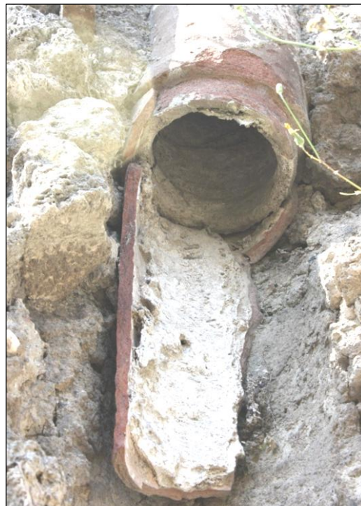
Figure 57B. The downpipe in the W wall of Room 93 contains thick calcareous incrustation. Photo: author, 2010.
