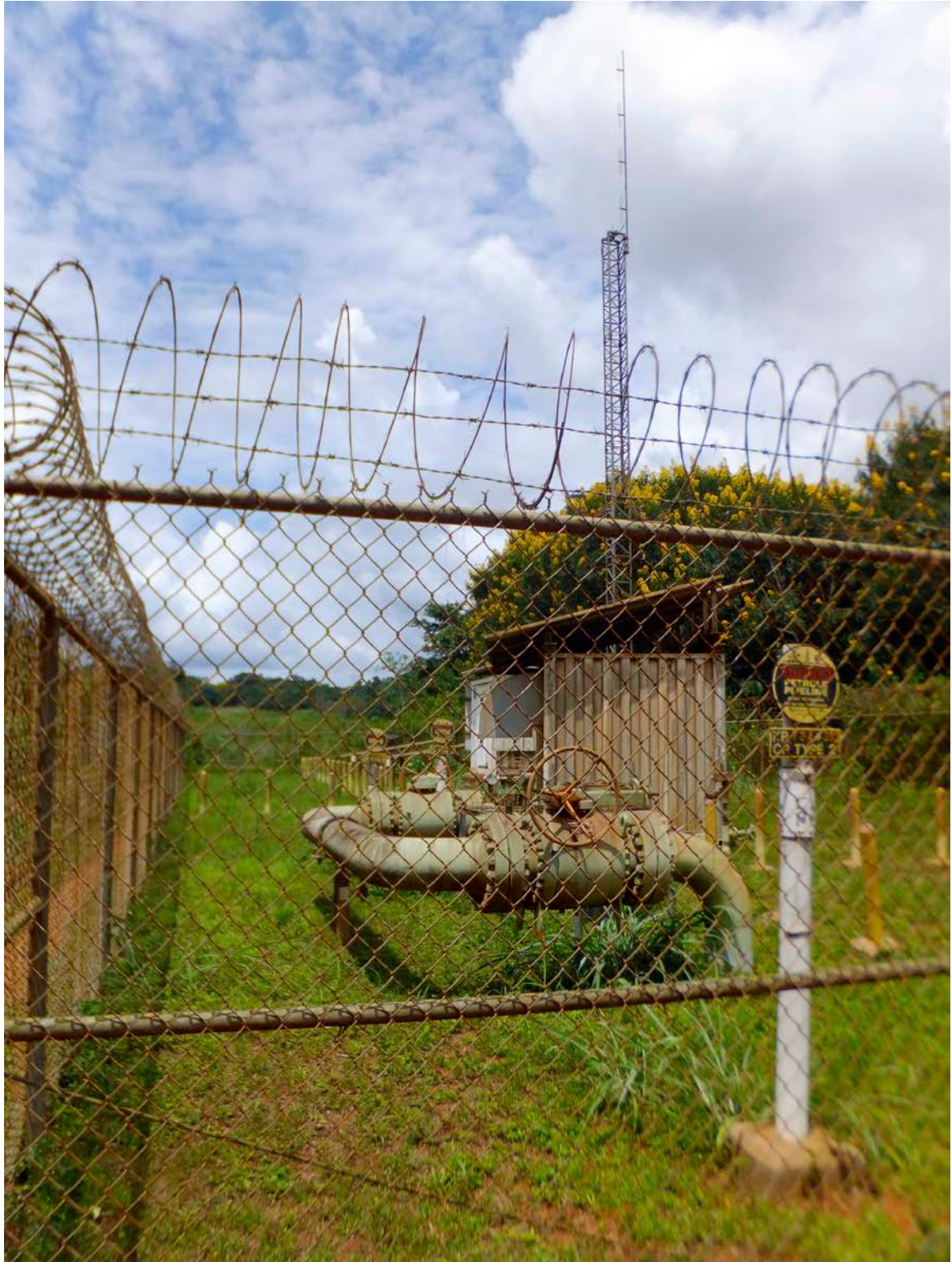
Figure 29. A fenced pipeline van station near Nanga.
