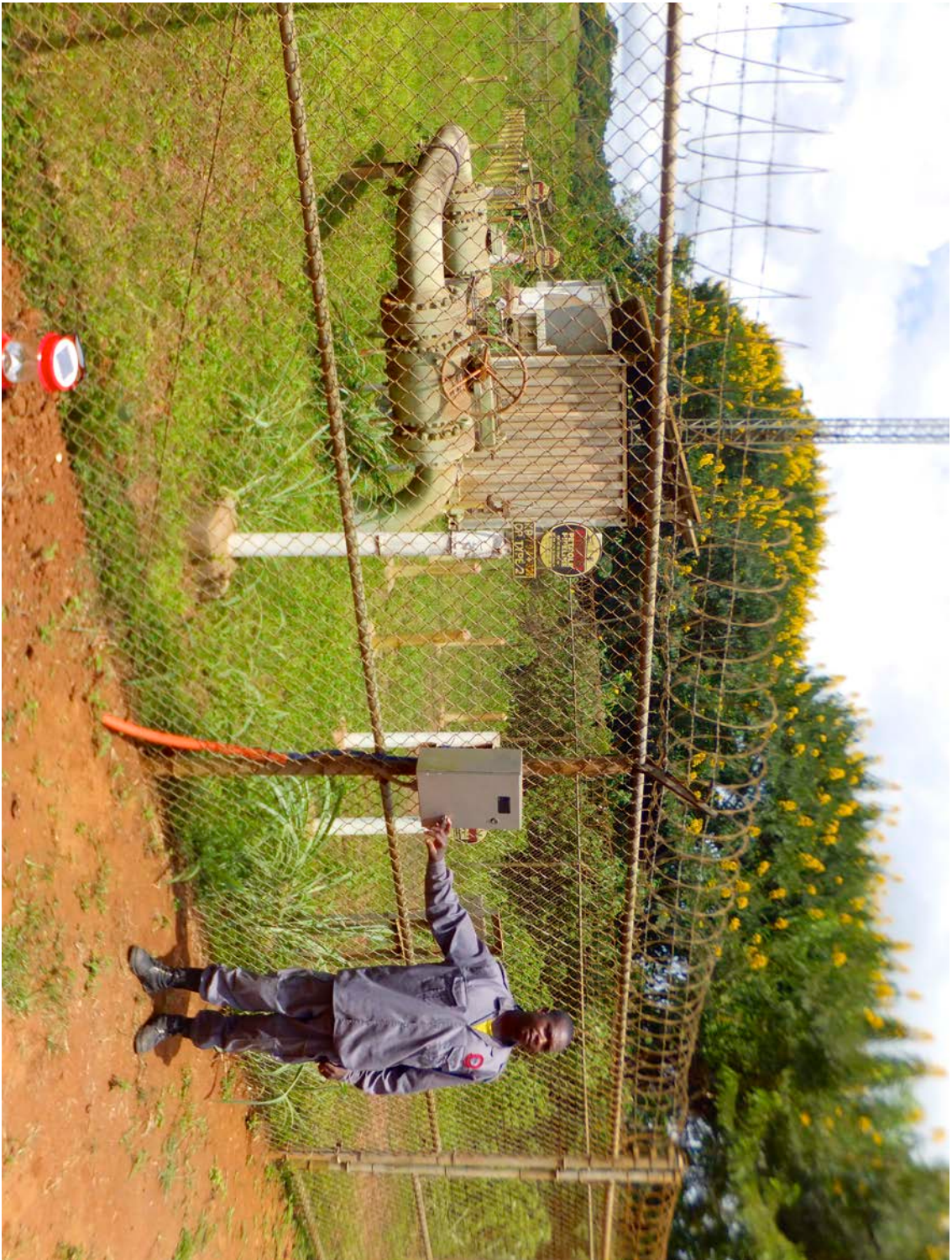
Figure 55. A COTCO security guard, standing in front of the pipeline valve station near Nanga.
