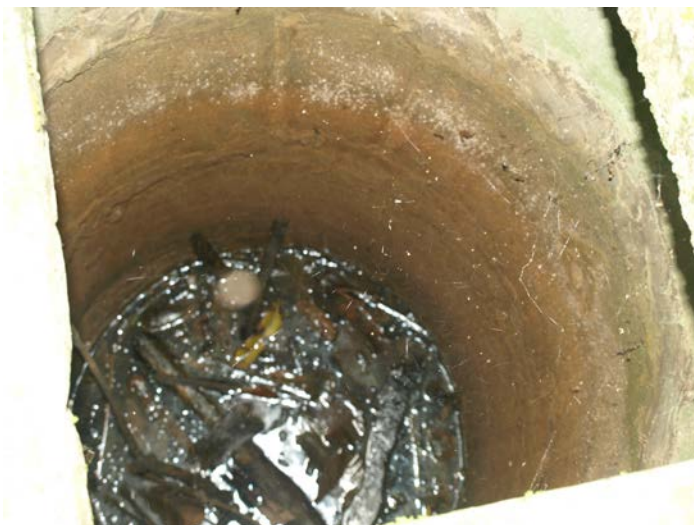
Figure 22. Looking down into a non-functioning well that was built by COTCO as reimbursement when a local borehole was destroyed during pipeline construction, Mpango.
