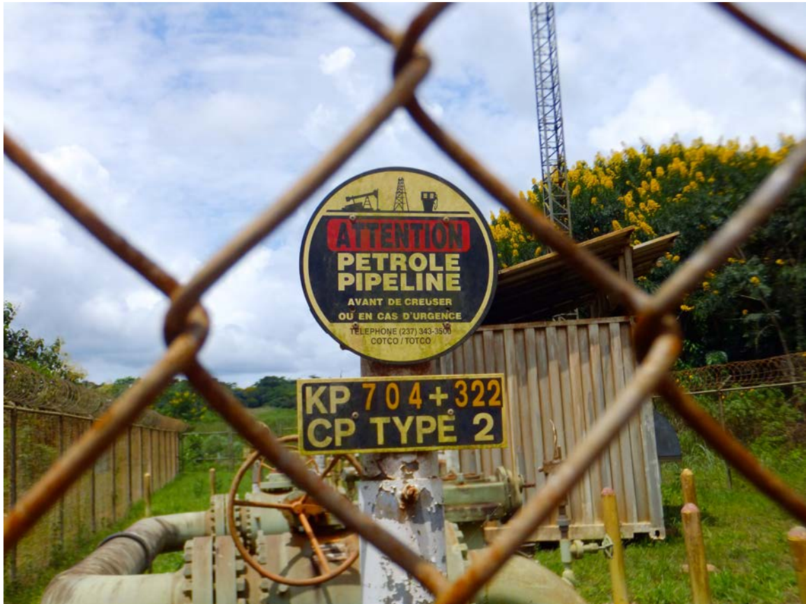
Figure 31. Looking inside the fenced aboveground pipeline valve station near Nanga.
