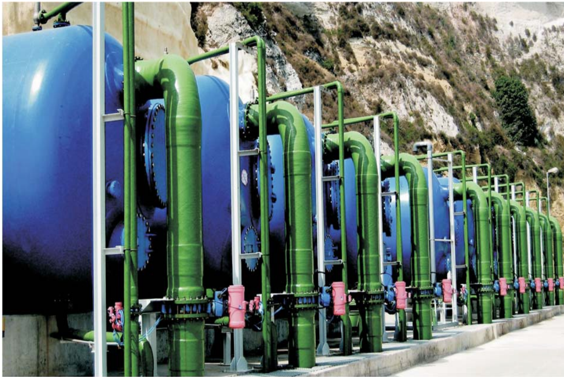
Water purifying plant
