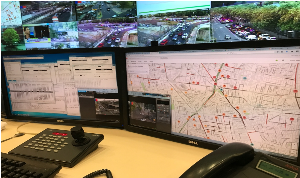
Figure 9 Control room operator desk-setting at the UOCT. Source: The picture was taken during one of my visits to the UOCT in December 2018.
