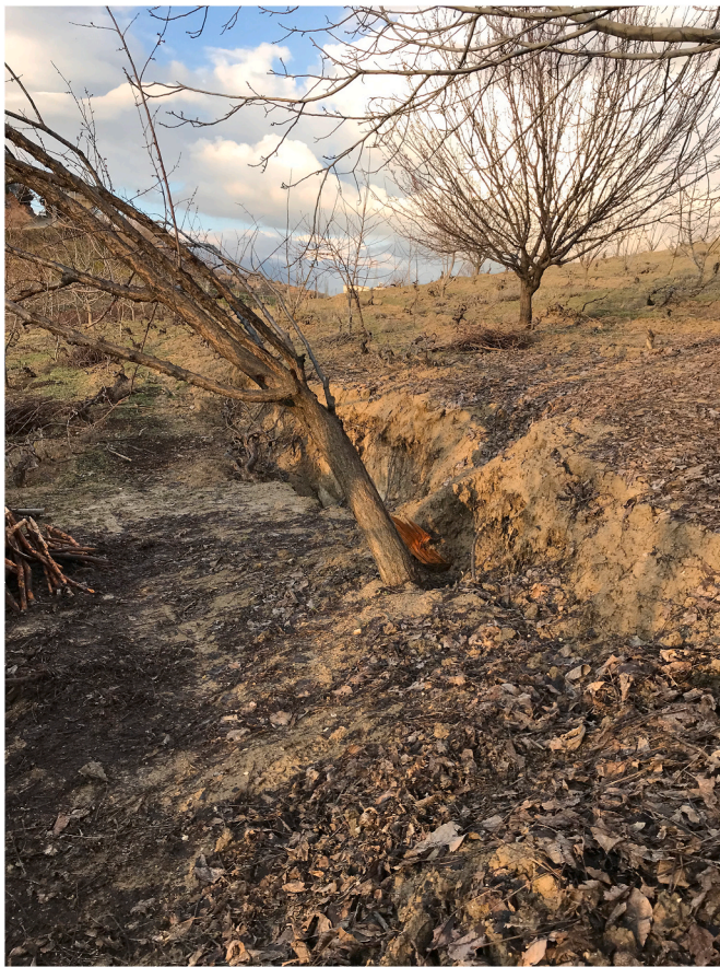
Fig. 14. Field photograph showing the fault rupture causing damage to the base of a tree located on the fault (location: 37 49 13.692 N; 37 41 7.2852 E; near Gölbasi).
