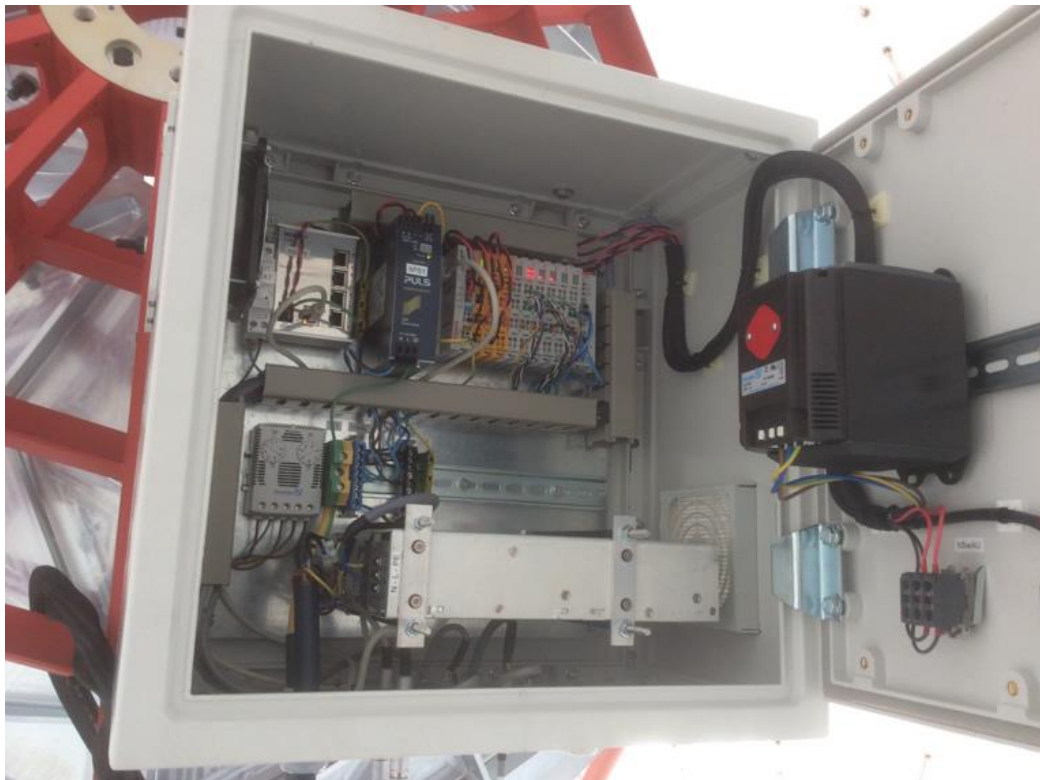
Fig. 5.4 Inside of the electrical cabinet on the rear of the secondary mirror structure, housing the camera power supplier.
