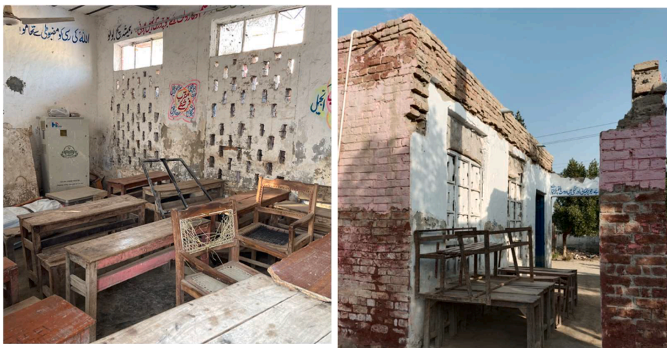
Fig. 4. School buildings after the floods (please print in colour).
