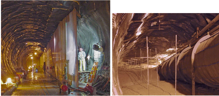
Figure 17: The NuMI Decay Pipe Tunnel. The left photograph shows the decay tunnel before the decay pipe was installed. The wall was the form for the concrete shielding and the worker shown was standing in the egress passage. The right photograph shows the installed decay pipe with concrete shielding being poured. The stiffening ribs around the pipe are also visible as well as the copper cooling lines running along the length of the pipe.
