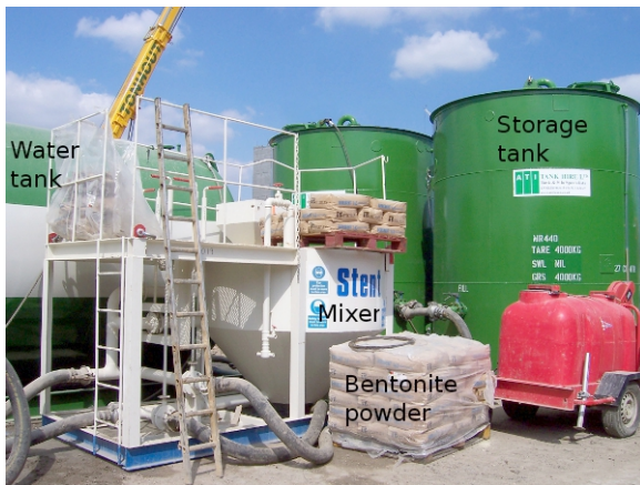
Figure 4.16: Bentonite mixing and storage equipment.
