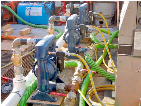
Figure 3.20: Three double-diaphragm pumps used in parallel. (Photograph courtesy of G. Goodhue.)
