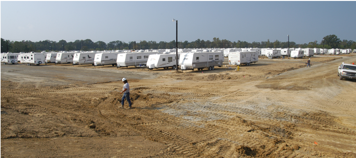
Figure S.1 FEMA trailer park under construction in Louisiana, late 2005. Photo by Marvin Nauman/FEMA.
