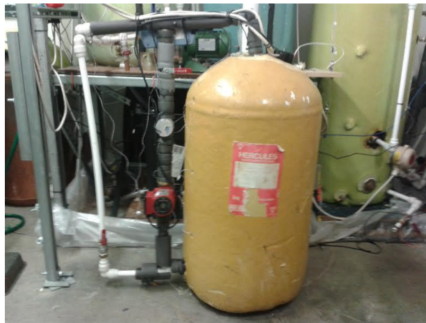
Figure 3-15 Photograph of tank from flat a retrofitted with destratification pump
