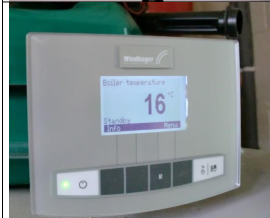
Figure 156: Heating controls on the domestic biomass boiler (TSB002).
