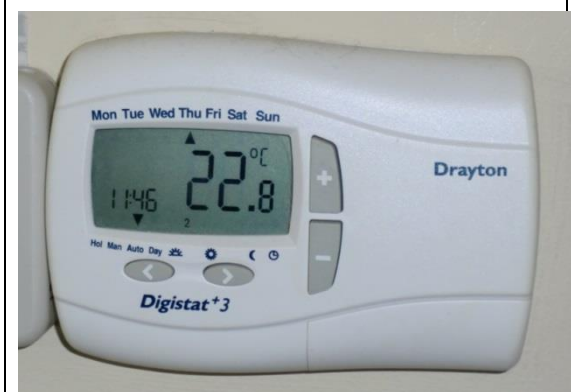
Figure 172: Case TSB110, heating programmer, room temperature indication 22.8 °C (13/10/2011) during POE walk-through.
