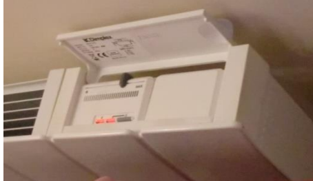
Figure 203: Storage heaters controls.
