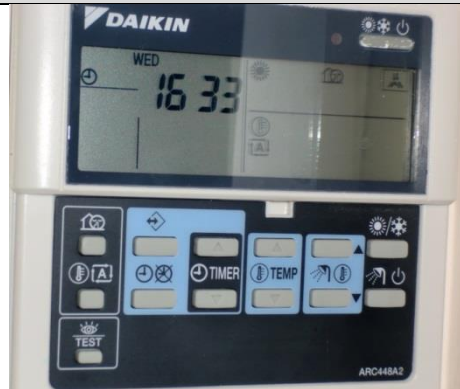
Figure 191: Programmer in ASHP system.
