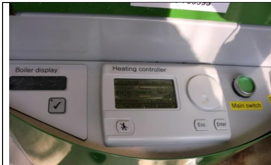
Figure 157: Heating controls on the domestic biomass boiler (TSB068,069).
