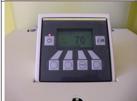
Figure 155: Heating controls on the domestic biomass boiler (TSB87).
