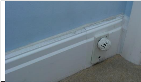
Figure 202: Thermo skirting heaters controls.
