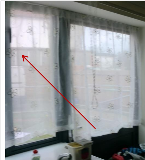
Figure 226: TSB033, kitchen window above the sink problem in operation due to the height of the handle position and reaching distance from the user.
