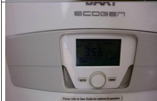
Figure 152: Heating controls on the Combined Heat and Power (Baxi ECOGEN micro-CHP) (TSB100).
