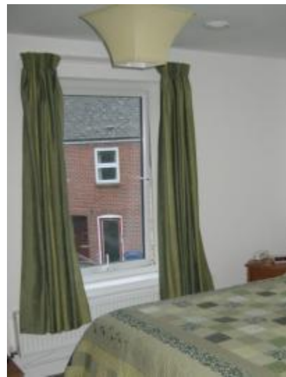
Figure 49: 'as built' triple glazed window, pivot/tilt opening type.
