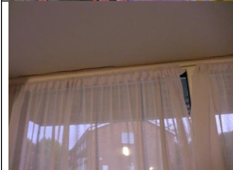
Figure 248: TSB113, cracks on the ceiling.
