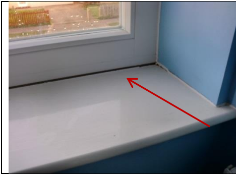
Figure 222: TSB 041, draughts from window due installation faults (gap between the window frame and board sill).
