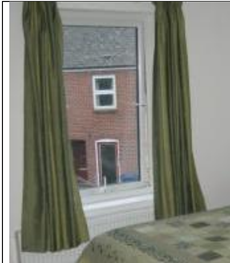
Figure 232: TSB054, operational problems in window opening due to one pane triple glazed window, pivot/tilt opening type increasing window weight and security issues due to lowering the window's sill plate.
