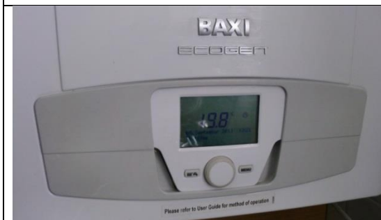
Figure 151: Heating controls on the Combined Heat and Power (Baxi ECOGEN micro-CHP) (TSB034).
