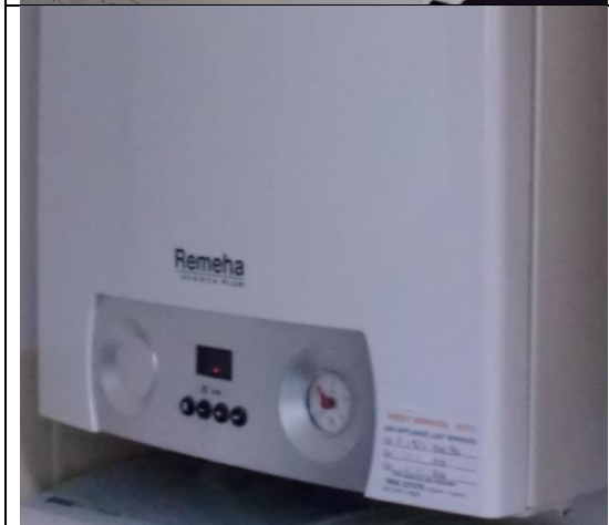
Figure 160: Controls on the gas boiler heating system.
