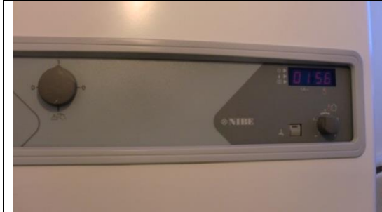
Figure 154: Heating controls on the Air Source Heat Pump boiler (ASHP) (TSB033).
