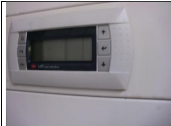
Figure 153: Heating controls on the Ground Source Heat Pump boiler (GSHP) (TSB076).
