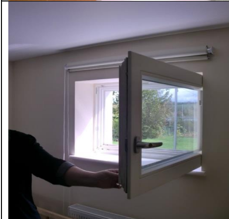
Figure 231: TSB036, operational problems in window opening due to increased size of bedroom window occupying large area of living space.
