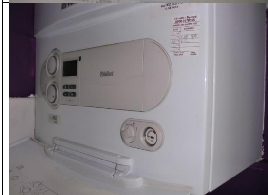
Figure 159: Controls on the gas boiler heating system.
