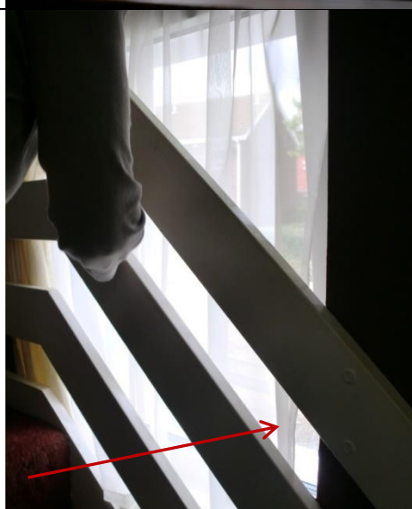
Figure 221: TSB110, problem in operation of the hall way window, as not only window handle cannot be reached by the user but also cannot be opened as blocked by the staircase rail.
