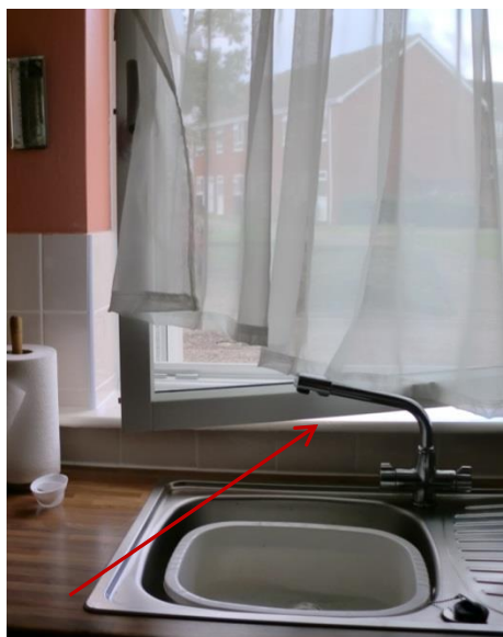
Figure 220: TSB110, kitchen window above the sink problem in operation window cannot be fully opened as blocked by the sink tap.
