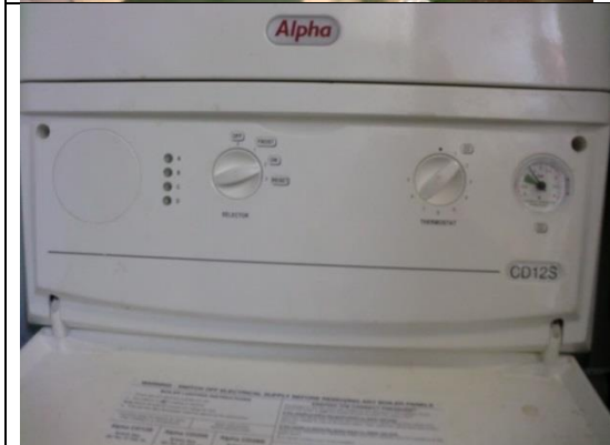
Figure 158: Controls on the gas boiler heating system.
