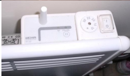
Figure 204: Storage heaters controls.
