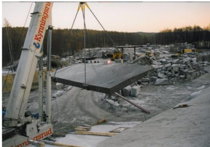
Figure 4: Granite wall on the move
