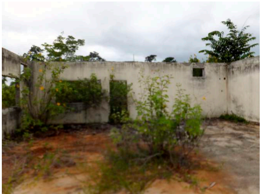
Figure 2. Another abandoned building, former pipeline work camp, outside Nanga (Amber Murrey)
