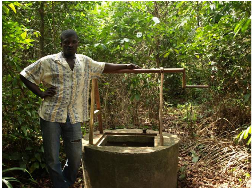
Figure 7. Non-functioning well that was built by COTCO as reimbursement when a borehole was destroyed during pipeline construction, Mpango (Amber Murrey)
