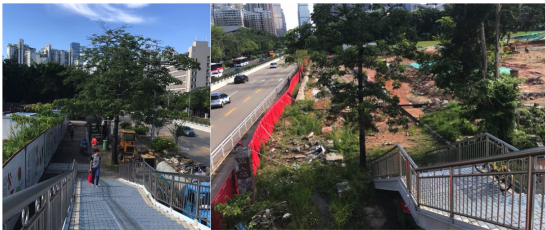
Figure 5.3 Construction sites narrowing pedestrian footpaths and creating walking obstacles
