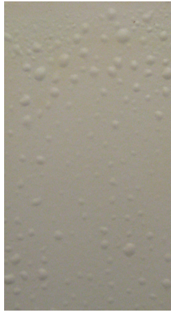
Figure 2.6 - Blistering on coated panel
