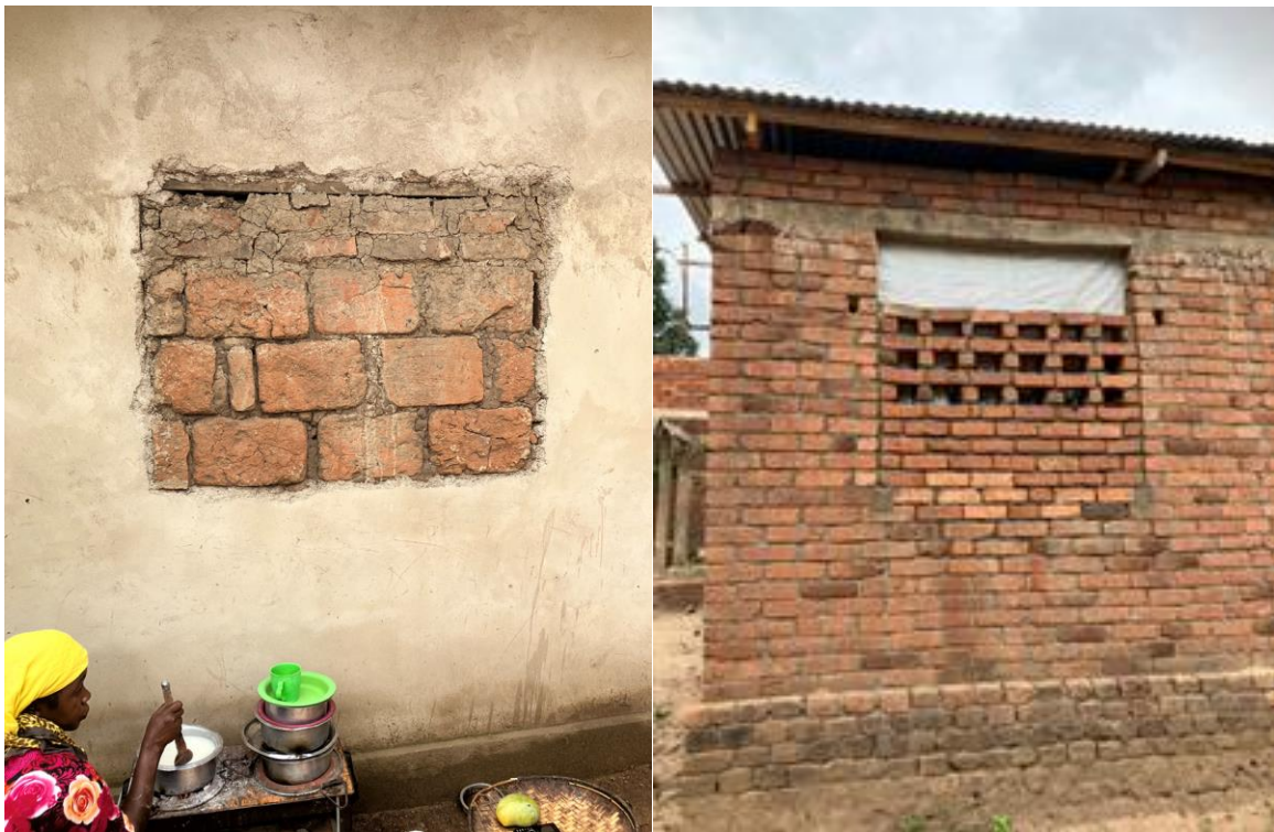
Figure 5 (a and b). Completely or partially blocked windows in the Kilombero Valley. Photos by the authors.
