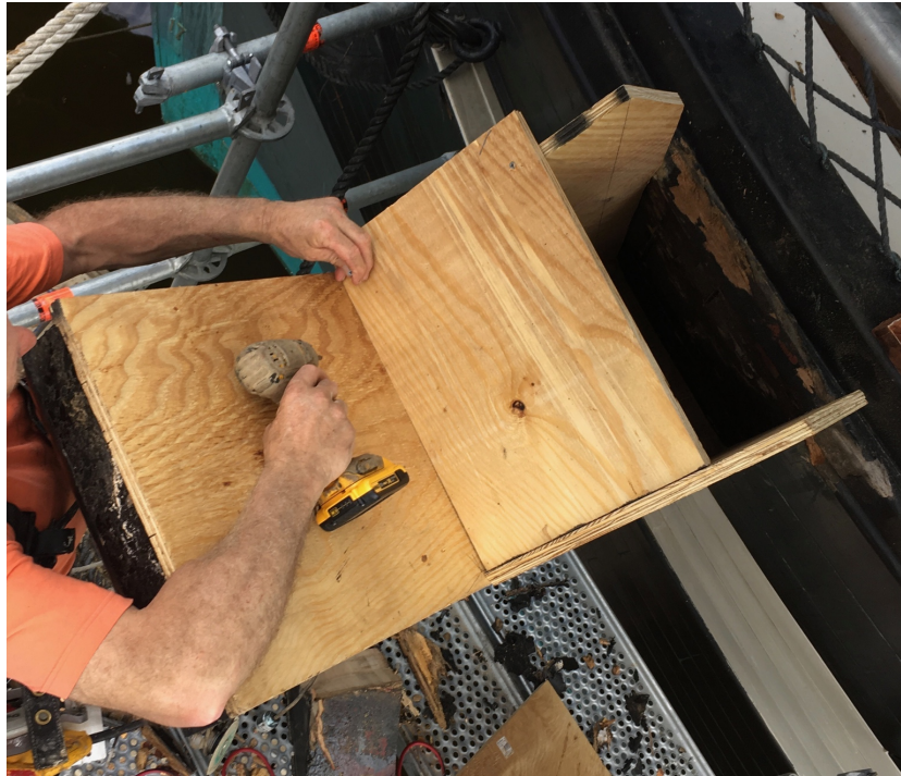
Figure 43: Harvey creates a template for the port cat-head by building it in place
