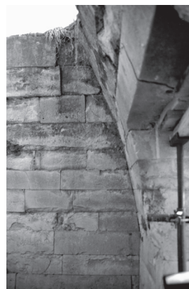
Figure 8 (above): Krannon, chamber tomb, detail of the upper part of the walls of the chamber.
