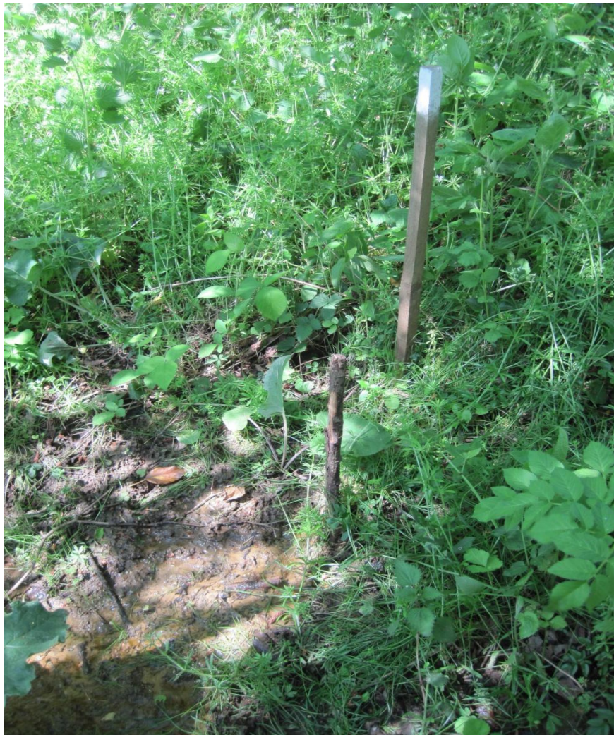
Figure 7 Stakes marking the changing extent of an embankment leak (note muddy area to left of stake)
