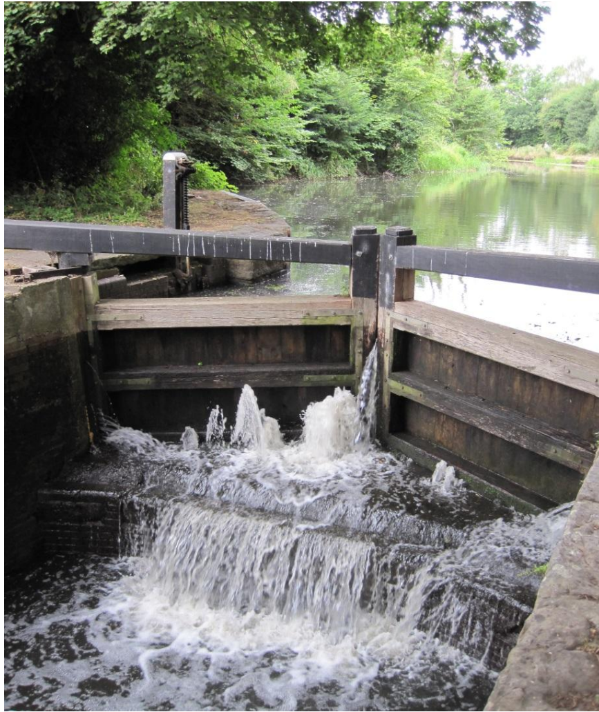
Figure 6 Leaking lock on the Basingstoke Canal
