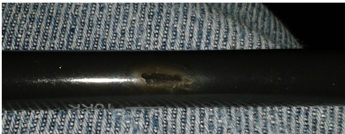
Fig. 3.23: Willow HTE 152 resistor rated at 48 kV. It was much more durable than the planar SLIM-MOX resistor, however after extended operation it started sparking from its surface (see burn mark in centre), which led to the use of three resistors in parallel, see Figure 3.24
