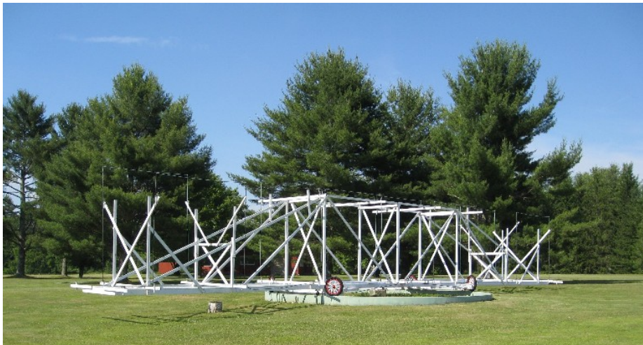
(a) A full-size replica of “Jansky’s merry-go-round”, a rotating antenna designed to measure 20.5MHz interference sources which could degrade transatlantic voice communications. It was with an array like this that Jansky first detected extra-terrestrial radio emissions.
