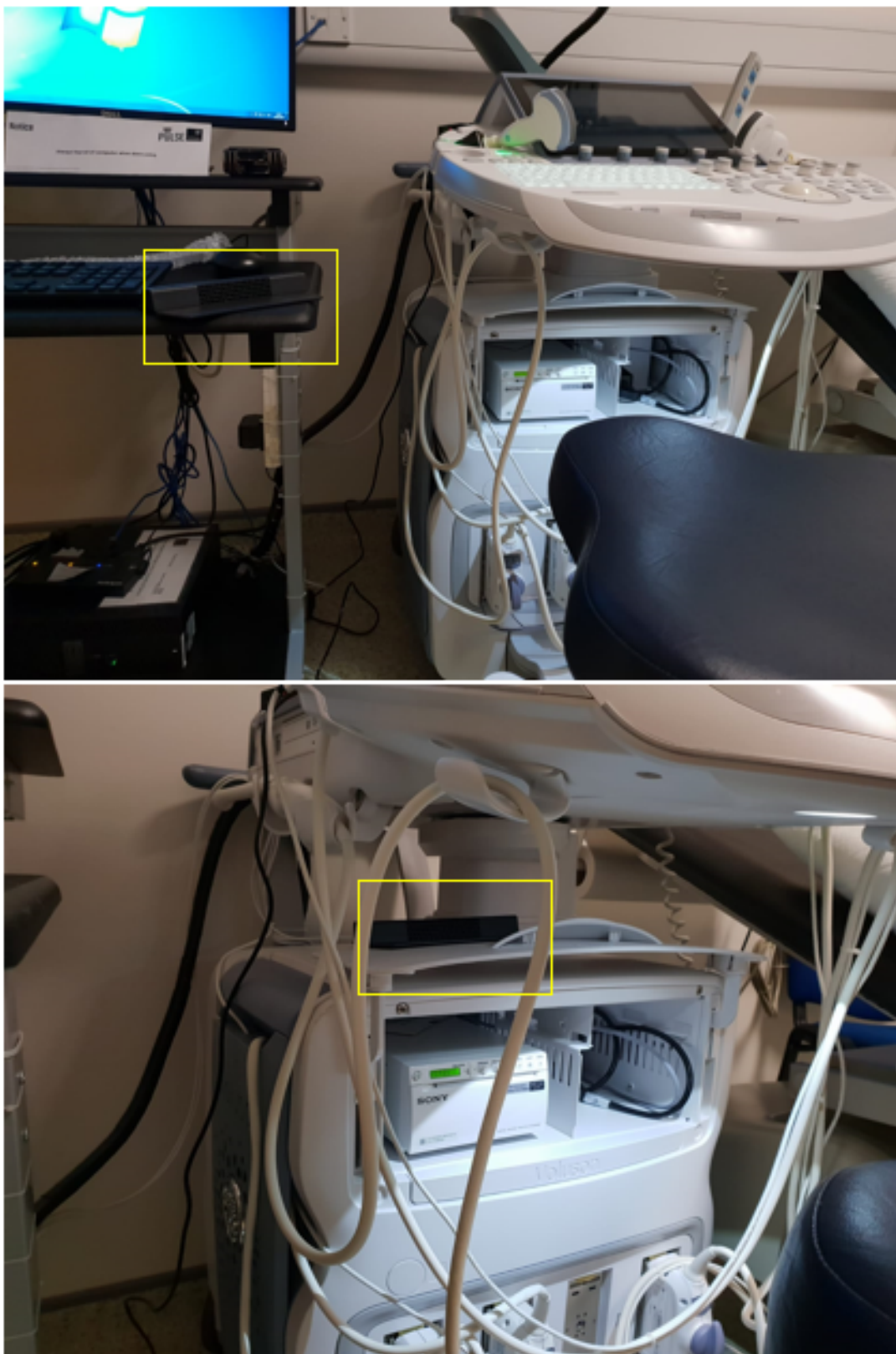
Figure 3.15: How a boundary microphone (such as the PCC160) could be installed in the scan room.
