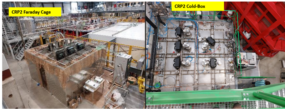
Figure 4.35. Left: TDE readout chain installed in the Faraday cage. Right: cold box setup for the CRP-2 tests in July 2022.
