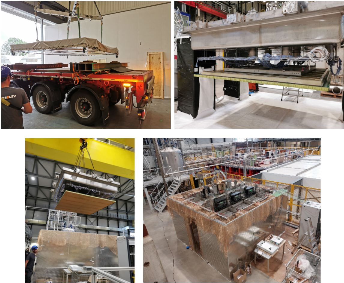
Figure 3.40. Top left: CRP-2 inside the transport box is being loaded to a truck for the transport to EHN1. Top right: at EHN1, CPR-2 is attached to the cold box roof and raised to the final height. Bottom Left: the cold box roof with the attached CRP-2 is on its way to the Faraday cage. Bottom Right: the cold box roof positioned at its final position on the Faraday cage room.
