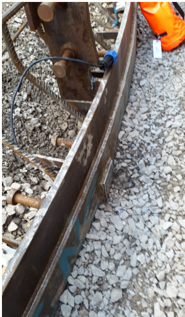
(c) Stroud cell in leading edge prior to concrete wall pour, see Figure 2.10 for layout.
