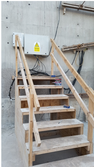
(c) Control unit on wall after wall is cast and prior to caisson sinking
