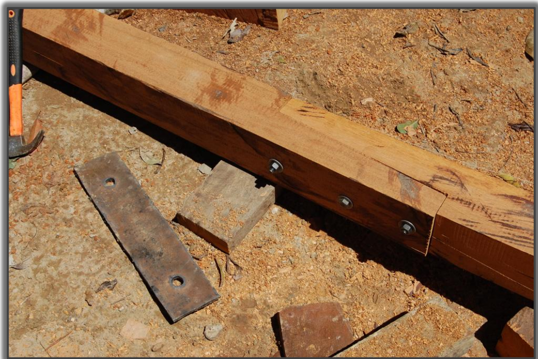
Figure 42: Support tower joint, with unused reinforcing plate
