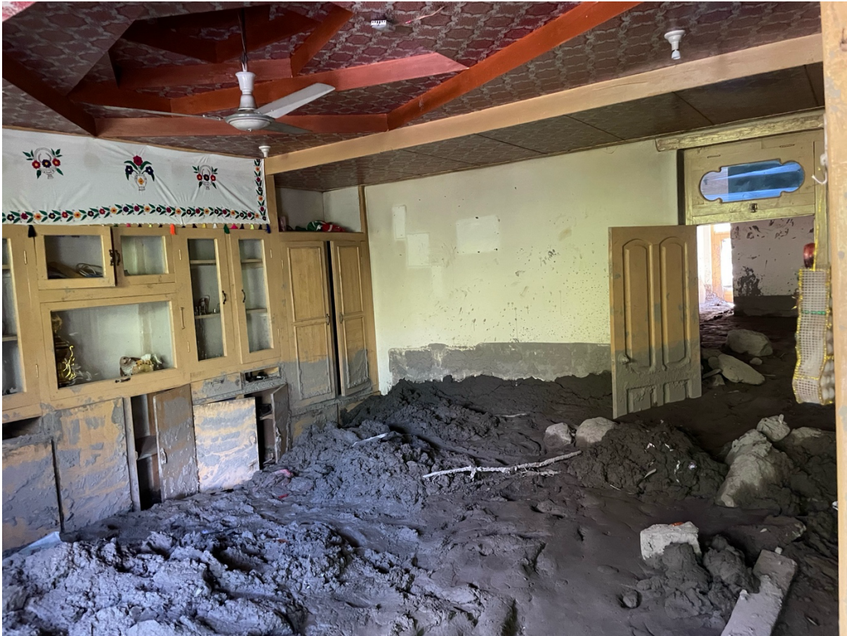
Figure 03: A house destroyed by floods in Chitral in 2022, captured by the author.
