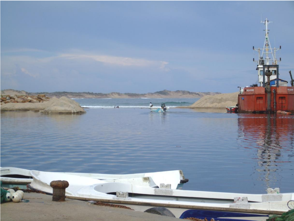
Figure 20. The inlet at the Kirinda harbour; despite constant dredging (right), only smaller sized boats are able to navigate through its narrow passageway.
