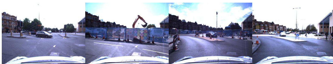
Figure 3.2: Significant road works were encountered over the data collection period. Each of the above images is from the same place (note the building on the left is visible in all images). In this example, the road network was altered to change the flow of traffic. Our system automatically updates its map representation when it detects change in the environment, including structural change.
