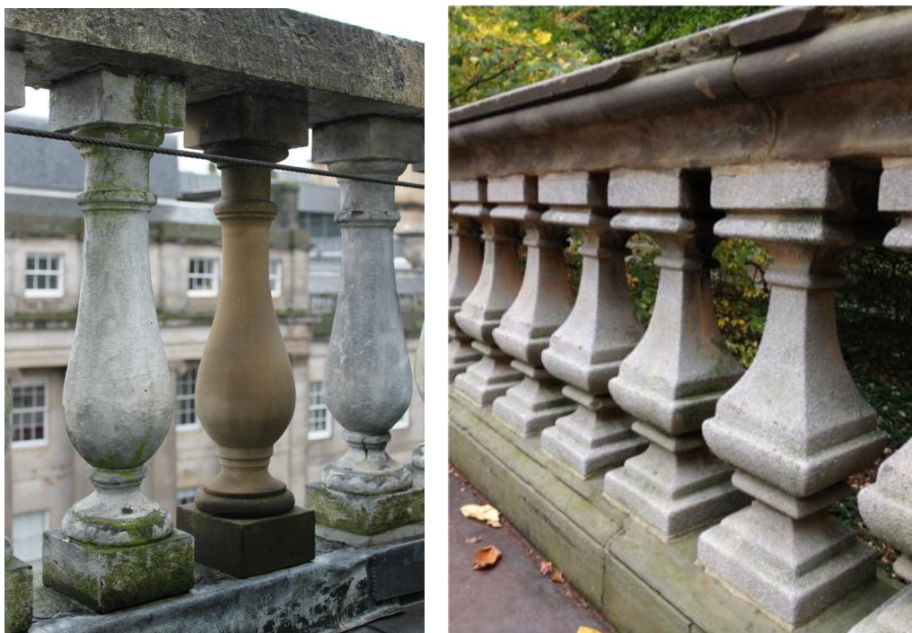
Left: Biological decay leading to replacement of sandstone baluster (2 Waterloo Place, Edinburgh), Right: Colonisation of cornice and plinth above and below recently cleaned brownstone balusters (Cedar Hill Bridge, Central Park, New York)
