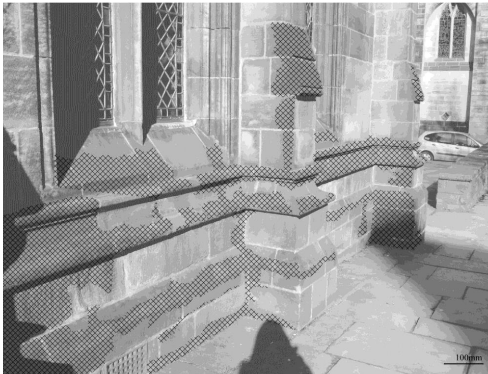
Figure 88: Patchy algal greening, eastern facade, Sheffield Cathedral
