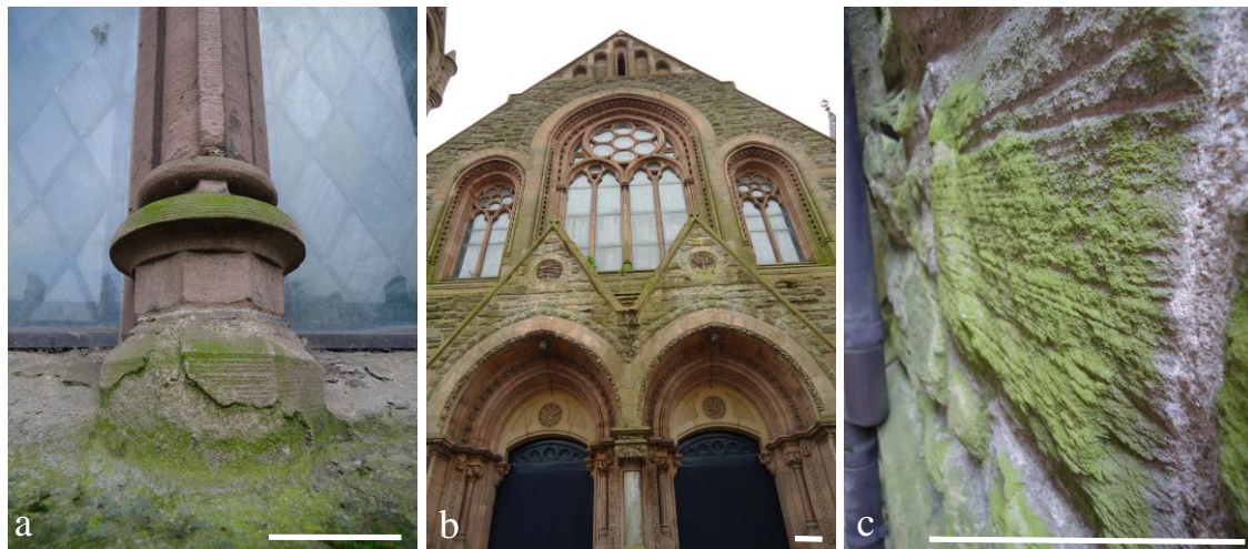
a. Heavy colonisation on windowsill associated with spalling surface crusts, b. General greening of front façade, c. dense biofilm development on ‘rusticated’ stone surfaces in a semi-sheltered location, northern façade. (Scale: 30cm)
