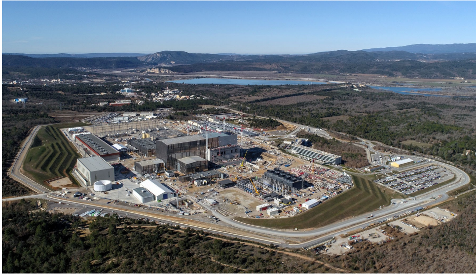
Figure 1.2.2: An ITER construction site photo in the south of France. This photo was taken in February 2020. Reproduced with permission from [67].
