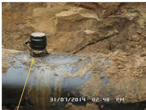
Close-up: Illegal fitting on 28" Trans Niger Pipeline at Ekpoko. Picture was taken during Joint Investigation of 31st July 2014.
