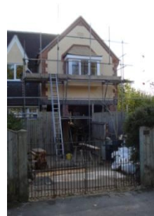
Exciting improvements Expensive repair
