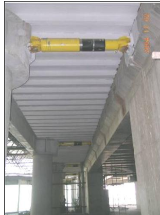
Figure 2.14. FVDs Linking Columns of Different Buildings to Eliminate Pounding in the Shanghai Shimao International Plaza (Lu, Gong, Weng, & Ren 2007)
