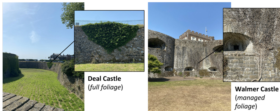
Fig. 2. The sections of wall and patches of ivy studied at Deal Castle (left) and Walmer Castle (right). Both walls are orientated towards the northeast, and are comparable in age, material, and design.
