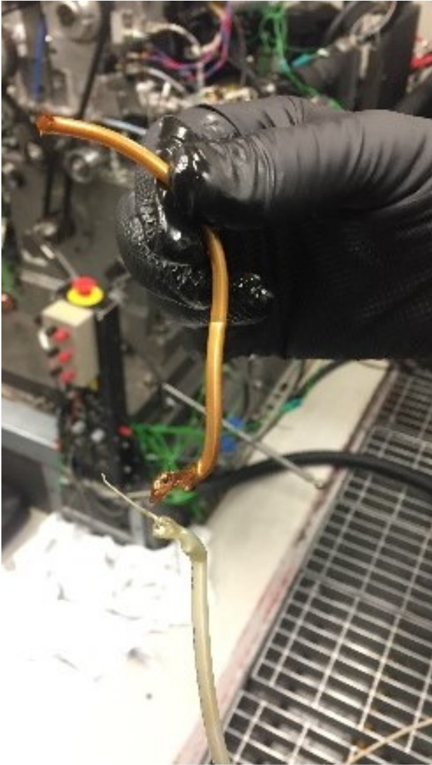
(a) Pipe failures (melted and detached)
