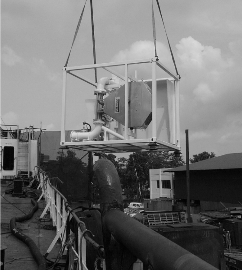
Figure 2. Half-container size skid can be swapped off the bunker barge for calibration or maintenance.
