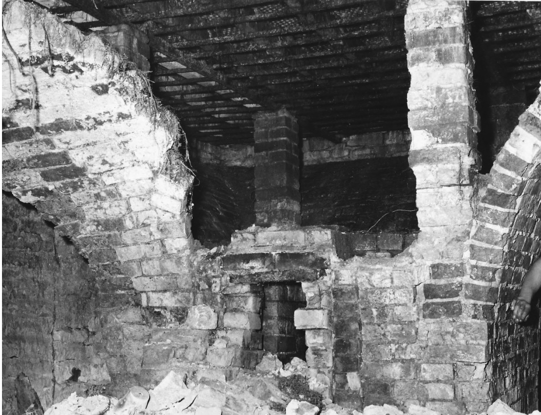
Figure 6 - Mid-nineteenth century corn drying kiln at the King's Mill, Stamford during demolition. Reproduced by kind permission of the Rutland & Stamford Mercury .
