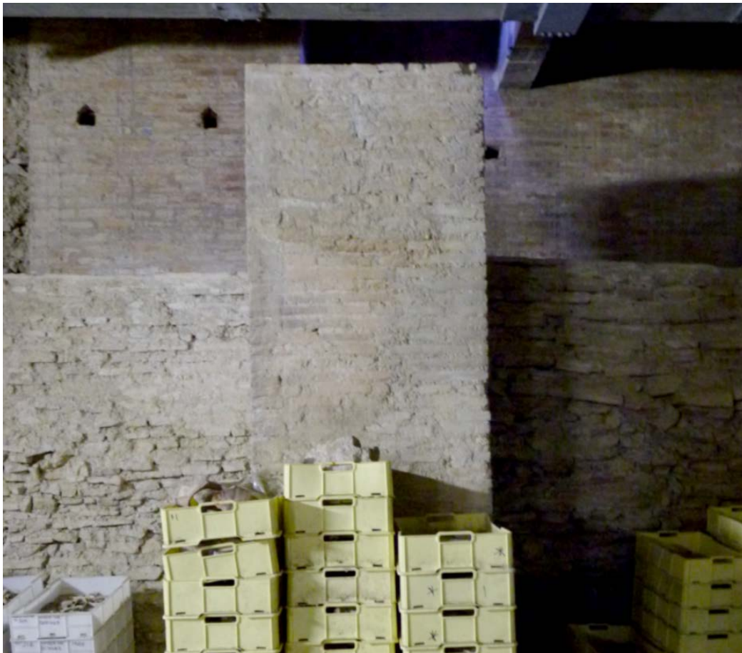
Fig. 3.12. West face of surveyed pier, showing the poor quality of the earlier structures incorporated into it (photo: Albuerne 2012).
