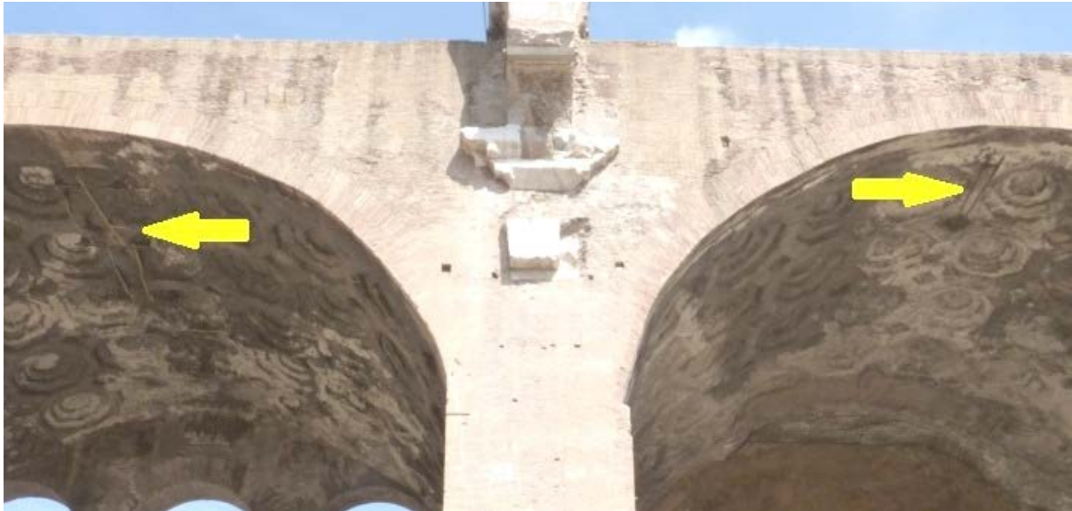
Fig. 6.7 West and central barrel vaults of the north nave of the Basilica of Maxentius showing visible repairs of existing crown cracks. Repairs dating from early 20 th century (photo: Albuerne 2011).
