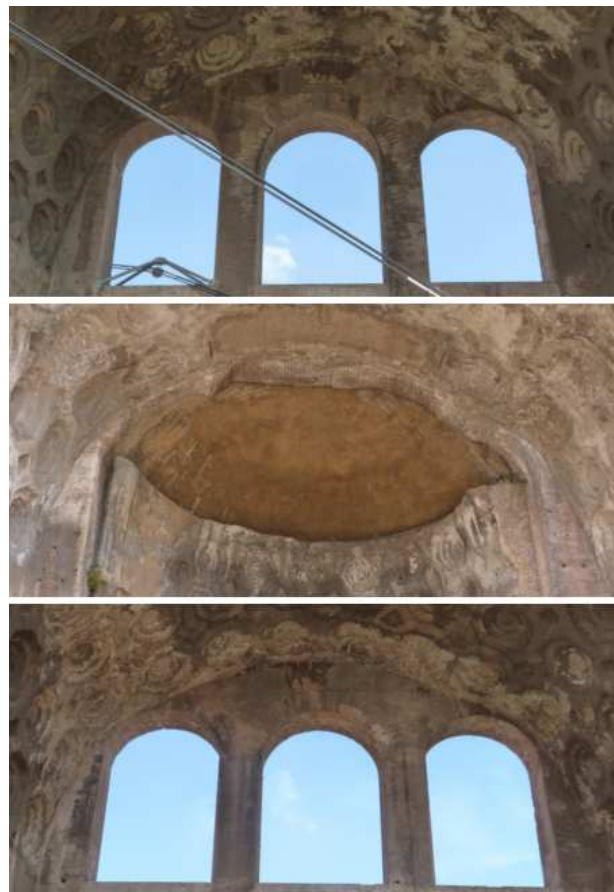
Fig. 2.5. Deformed profile of barrel vaults next to north façade. Left: west vault; right: east vault.
