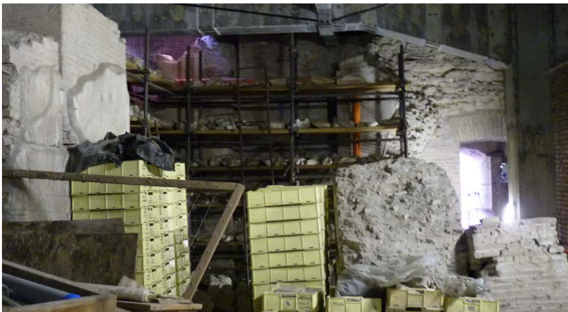
Fig. 3.14. Internal face of west façade, south nave, seen from inside the excavated basement (photo: Albuerne 2012) . A heavy duty shelf obstructs the view and access for a better survey.
