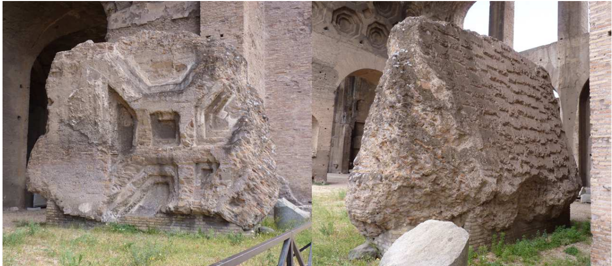
Fig. 2.14. Fragment A from the missing cross vaults of the Basilica of Maxentius: intrados (left) showing the coffering; and extrados (right) showing the traces of a tiled finish.
