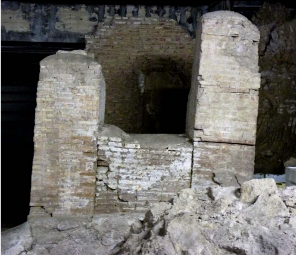
Fig. 3.7. Remains of Horrea Pipperataria, the building that occupied the site before the construction of the Basilica. These show signs of lateral load damage. Notice un-bonded behaviour at bipedales layers.
