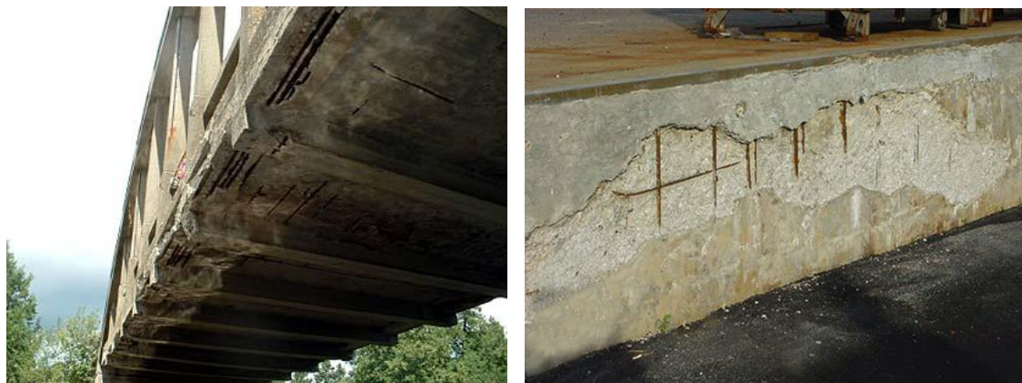
Figure 5.1. Images of steel corrosion in reinforce concrete.
