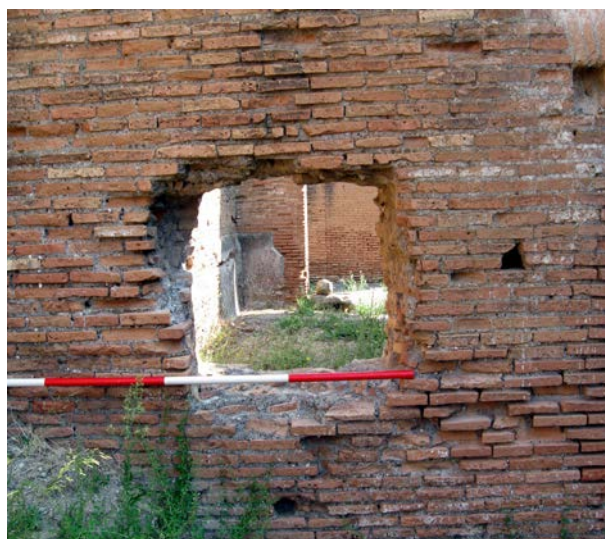
Figure 5.3: Hole in a wall in the Insula dell'Ercole Bambino with exposed core. Photograph by author.
