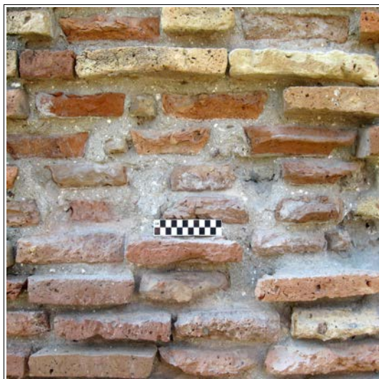
Figure 6.9. Very soft degrading mortar in Caseggiato del Larario. Scale =12 cm. Photograph by author.
