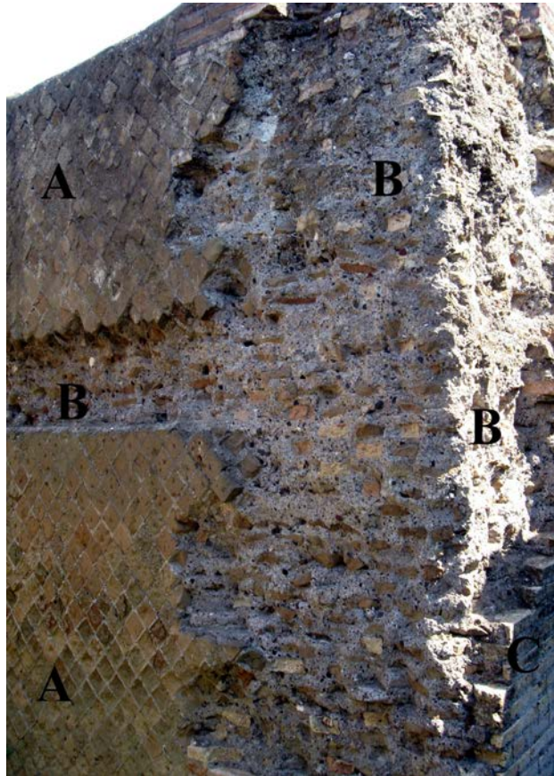
Figure 5.2: Edge of wall in the Casa a Giardino showing previous damage, intact tuff reticulate facing (A) and the exposed core (B). Photograph by author.
