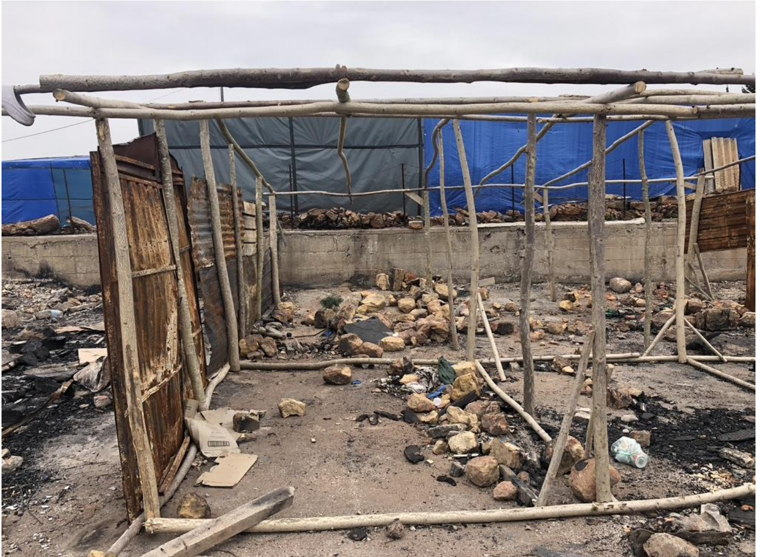
Figure 18 The frame of a house being rebuilt at the ex-cement factory, after the fire (photo by author)
