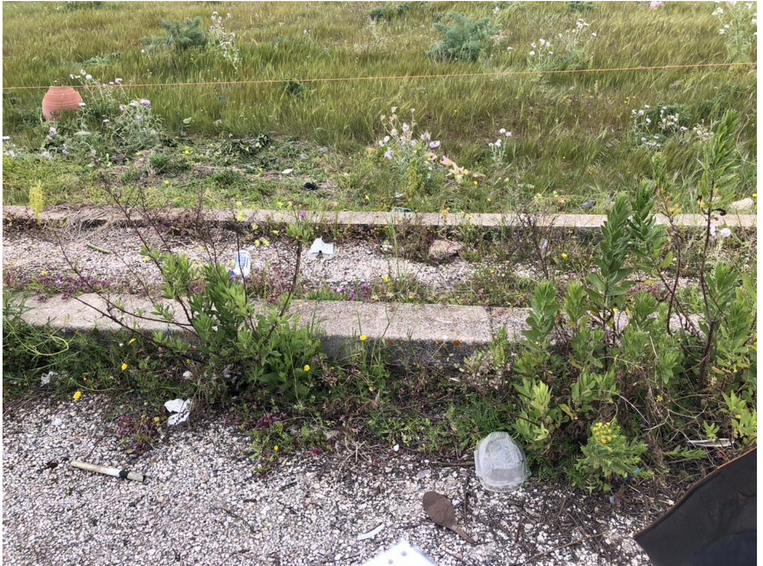
Figure 12 Unfinished sidewalk in Campobello (photo by author)
