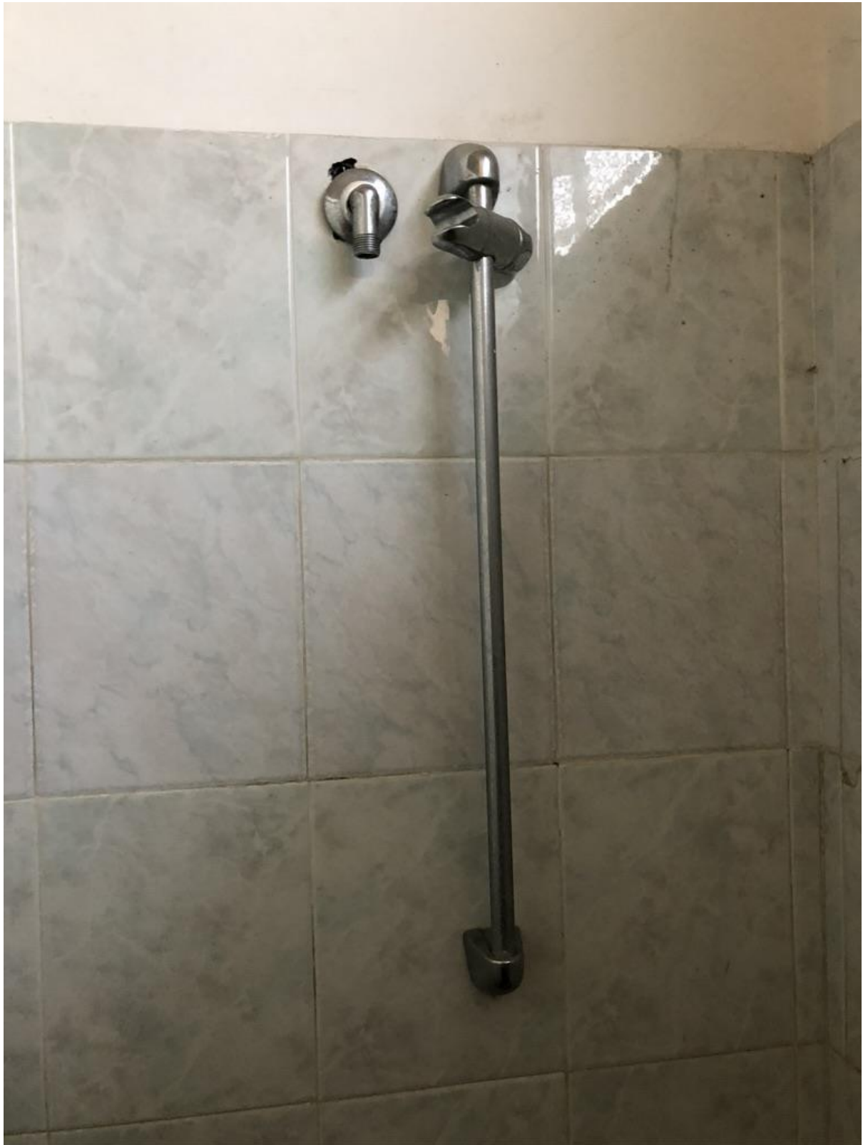
Figure 26 A broken shower in a reception centre (photo by author)
