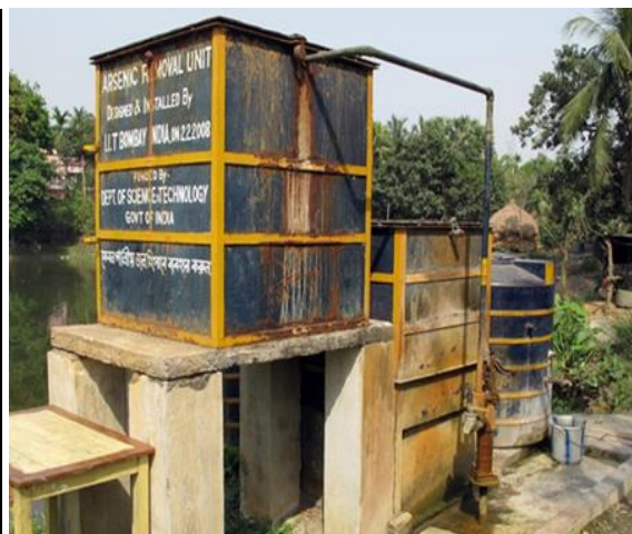
Photo 1.2 IITB with two tanks
