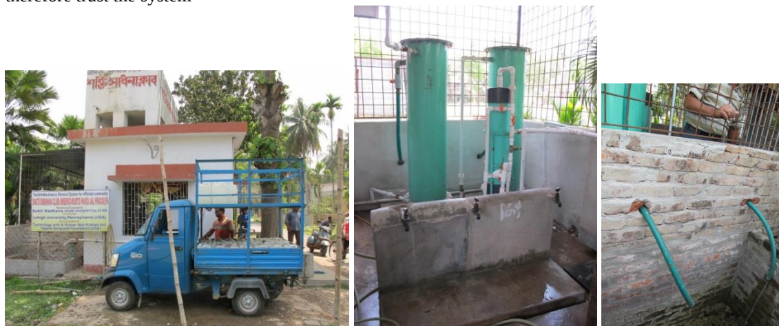
Photos: Small delivery truck parked beside the building that houses the BESU 3:1 filter. The middle filter photo is of the filter from the inside of the building, and the backwash exits out the hoses through the brick wall to a brick-lined hole beside the building.
