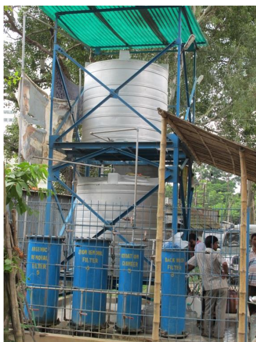
Photo 1.6 PalT/Harbr with an extra sand filter column used for backwashing
