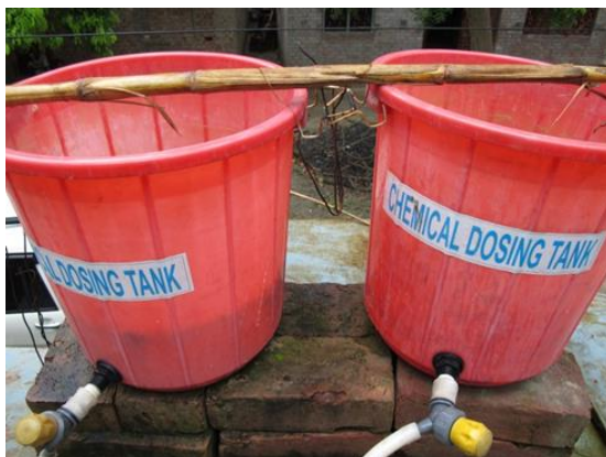
Photo 1.8 Chemical buckets onto of the filter
