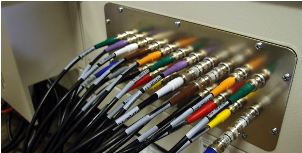
Figure 6.6: BNC cabling from multibeam receiver to HIPSR cabinets. Cables are colour coded for easier identification.
